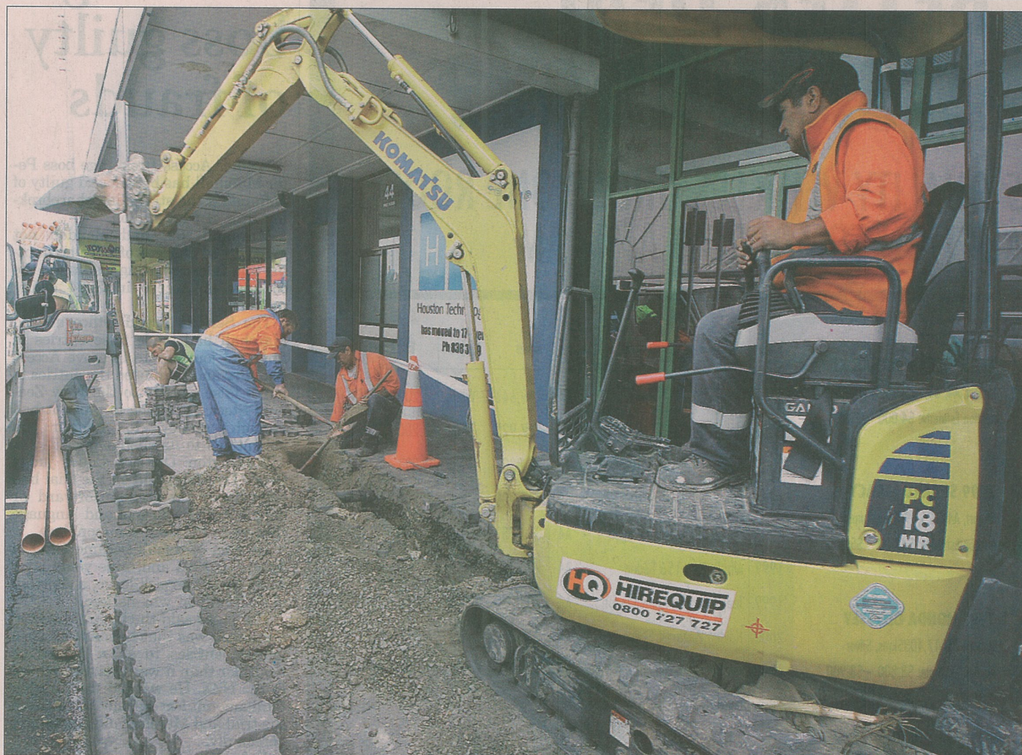
DIG IT: Workers dig trenches and lay pipes for Velocity to lay cables in future.
